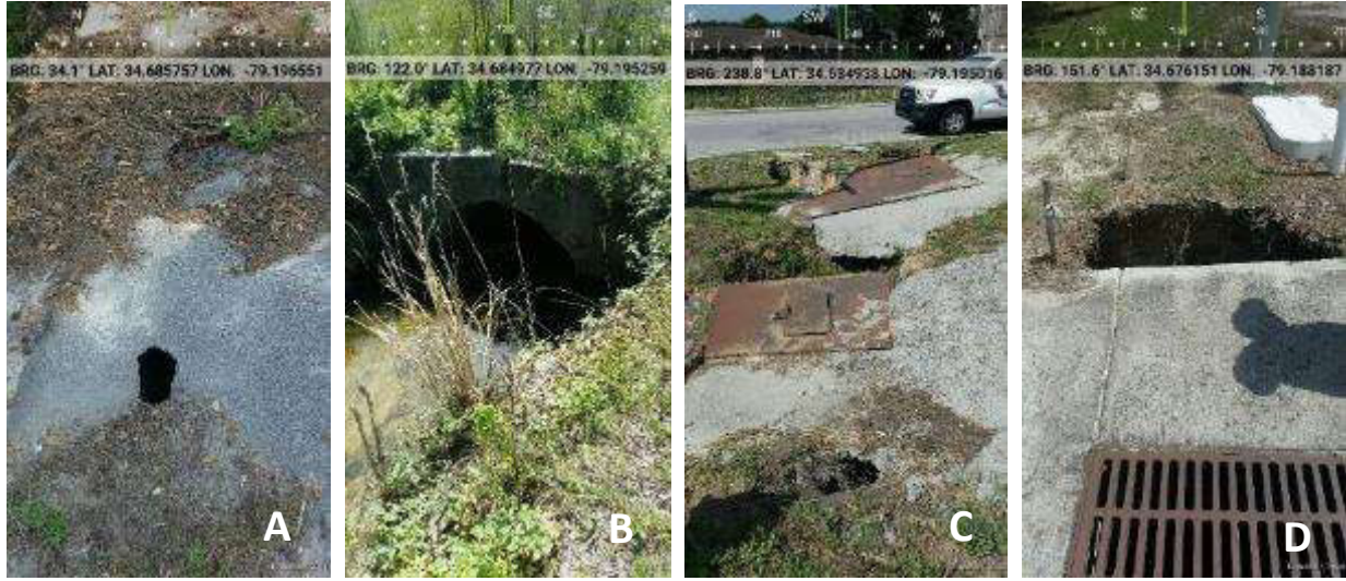
Images 1A-D. Observations of structural damage and possible improper installation along conveyance measures in short-term corridors.
