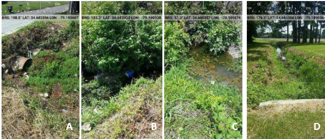
Images 2A-D. Observations of excess vegetation hindering the effectiveness of conveyance along the short-term corridors.
